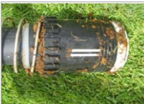
Figure 2. Sprinkler clogged by the scale
